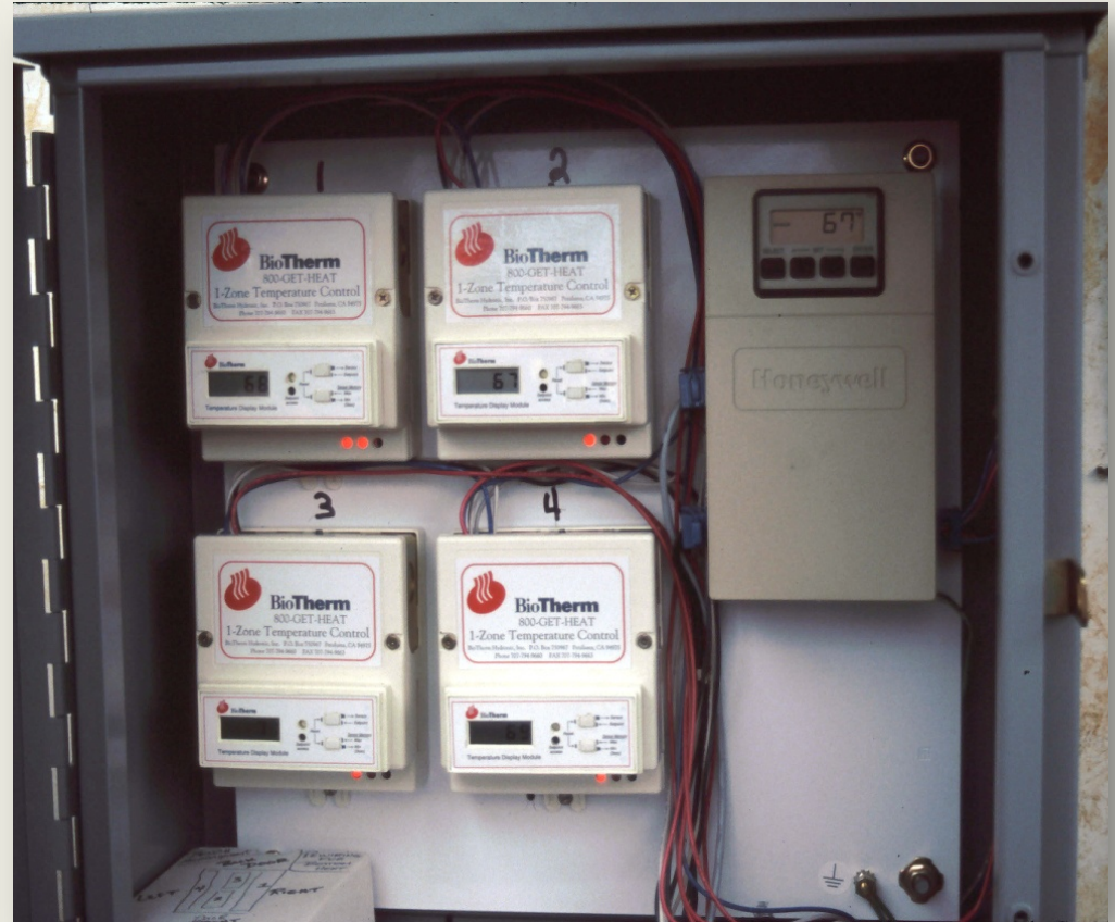
Temperature control unit
