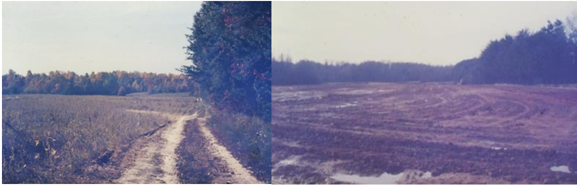
Figure 3. In the beginning: (left) Buds & Blooms Nursery, November 1983; (right) leveling and grading the former row cropped fields for containerized nursery production.
