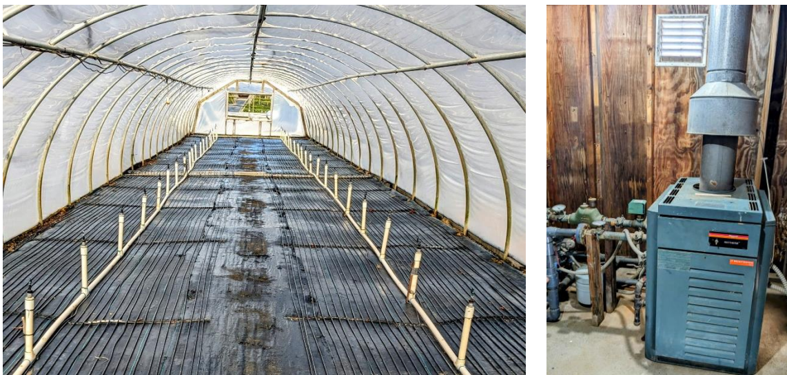
Figure 9. (left) BioTherm bottom heat, hot water tubing system for mist propagation, and (right) a Ray-Pac hot-water boiler.
